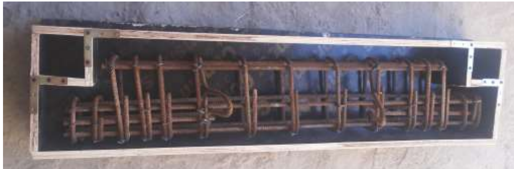
b. Typical molds and reinforcement of R.C. inverted dapped-end girder, without opening and strengthening.
