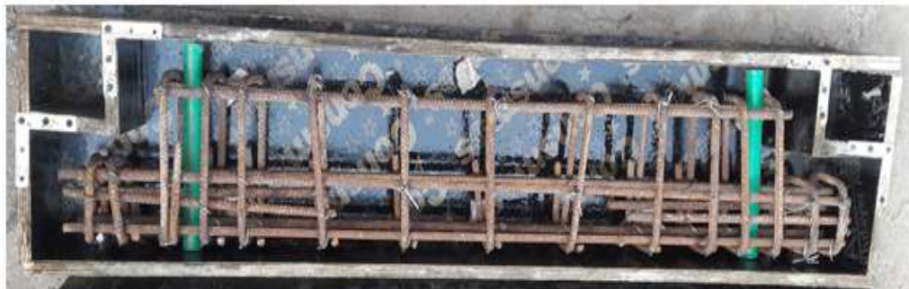
c. Typical molds and reinforcement of R.C. inverted dapped-end girder without opening with strengthening.
