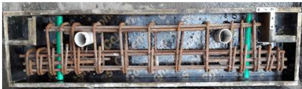
d. Typical mold and reinforcement of R.C. inverted dapped-end girder, with opening and strengthening.
