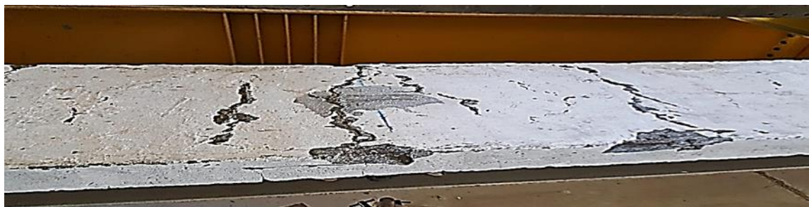
Fig. 11 The Mode of Failure of the Steel Girder (GR1) G1
