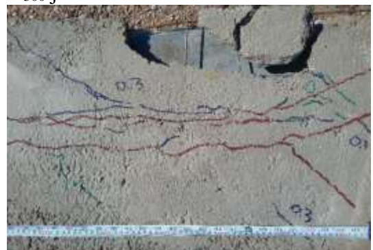
(c) Lateral crushing of concrete deck
