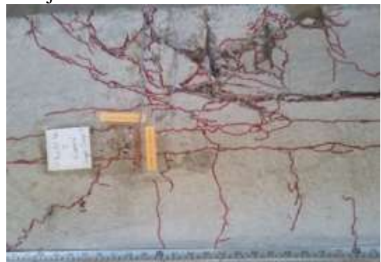
(c) Flexural cracks top view
