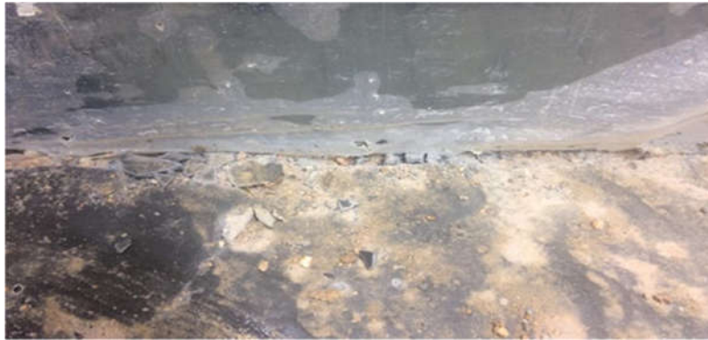
Fig .20 Broken sides of the layer treated by using 10%by volume of cement
