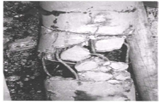
Figure 9: Pile damage at two lateral ground displacement during the 1964 Niigata earthquake [32]
