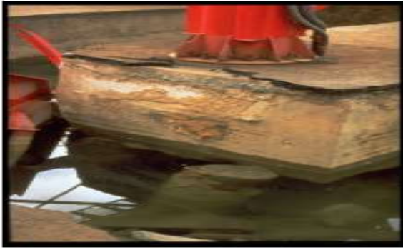
Figure 6: pile cap and failed pile supporting the Higashi-Kobe ferry pier [58]
