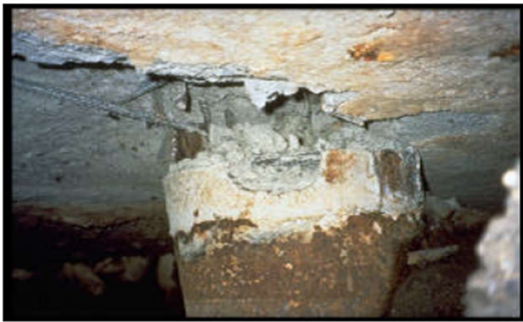
Figure 7: Failed piles and pile cap supporting the Higashi-Kobe ferry pier [58]
