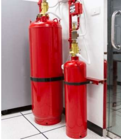
شكل 12: Novec 1230 Fire Suppression [33]2
